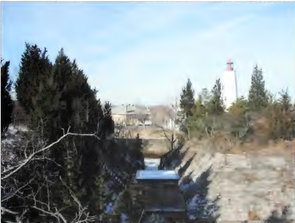
Figure 5.72. View looking northwest above mortar pit, the Mortar Battery. Woody vegetation greater than four-inches diameter should be removed from engineered slopes, and all woody trees and shrubs must not be allowed to grow upon, or within four-feet of a concrete structure or feature (Olmsted Center, January 2009).
